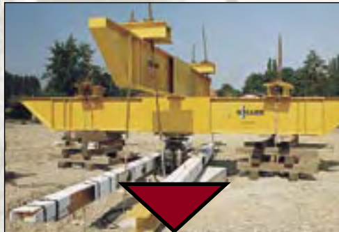
Load tests are a suitable option to verify the improvement of the soil
