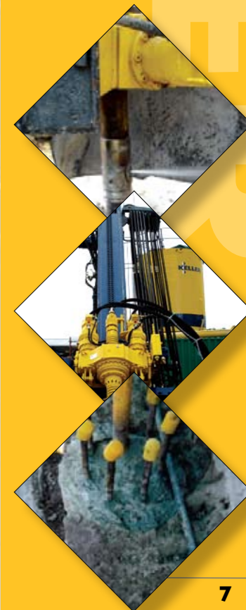
Top: Self Drilling jet grout monitor Middle: Drill head and mast configuration Bottom: Joint sealing between piles
