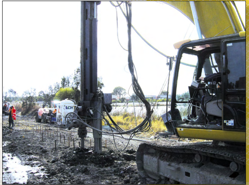
Column mixing for new rail track on deep soft clay, Newcastle NSW
